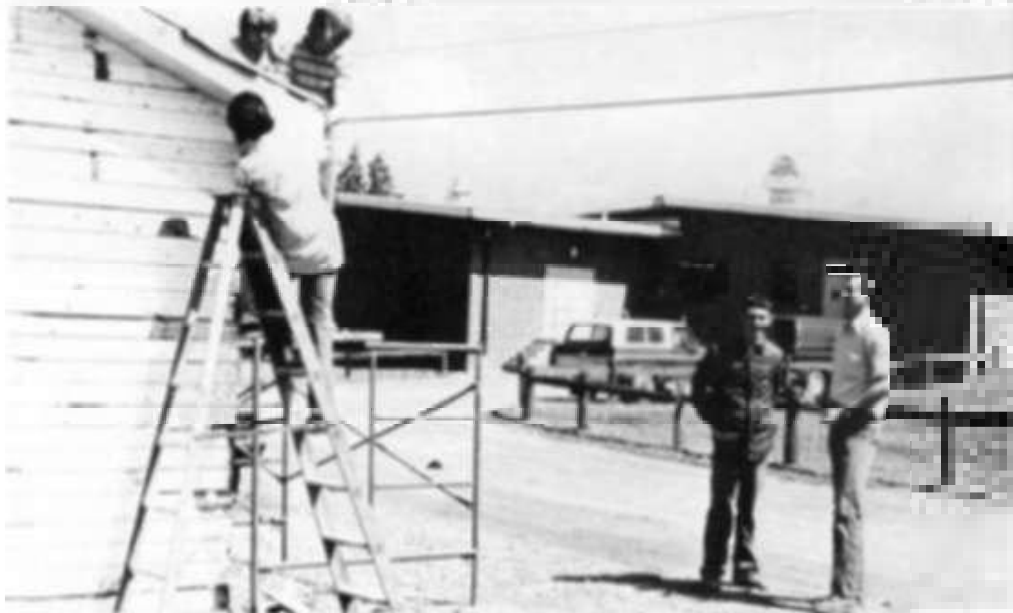
Above, Mr. Sam Taylor, Carpentry instructor, instructs his students about a building project. Working on the building are David Williams, James Neady, James, and standing on the ground are Clyde Perkins, junior, and Mr. Taylor with Kevin Hefner.
